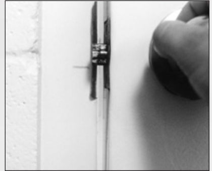
12. I also marked the position of the latch at the strike plate.
